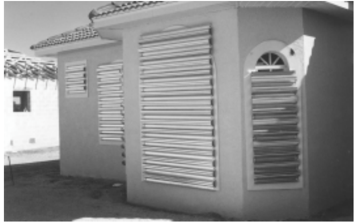
Storm Shutters (Opening Protection)
